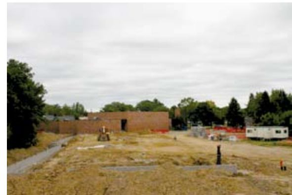
Foundation of the new expansion was completed in the second week of September 2006.
